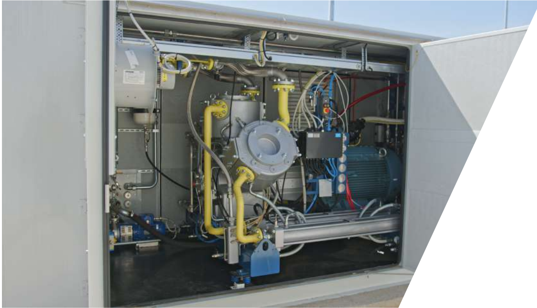
CNG Compressor and filling stations
